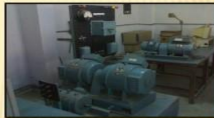
CONTROL SYSTEM LAB
