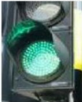
LED traffic lights
